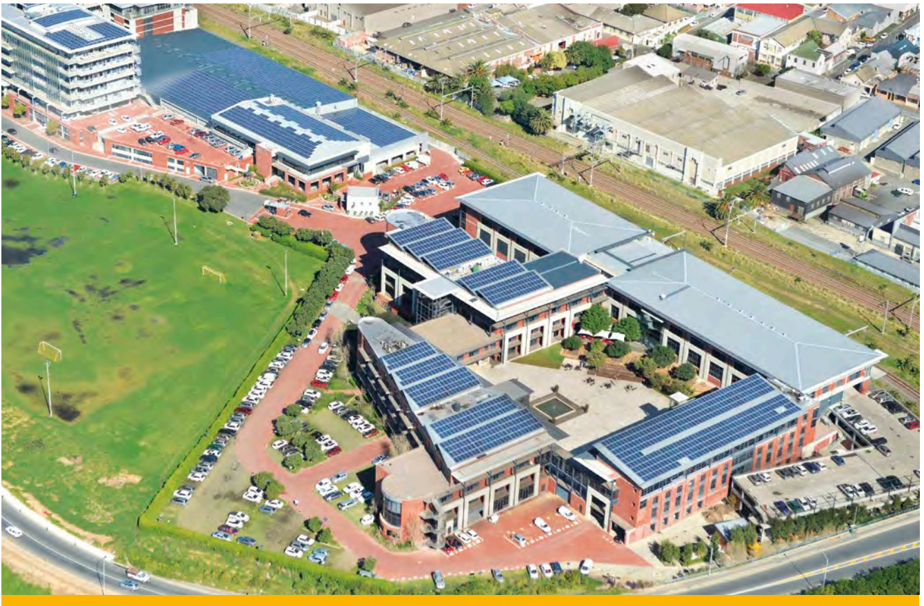
Grid-tied PV system at Black River Park. Photo credit: Bruce Sutherland, City of Cape Town.
