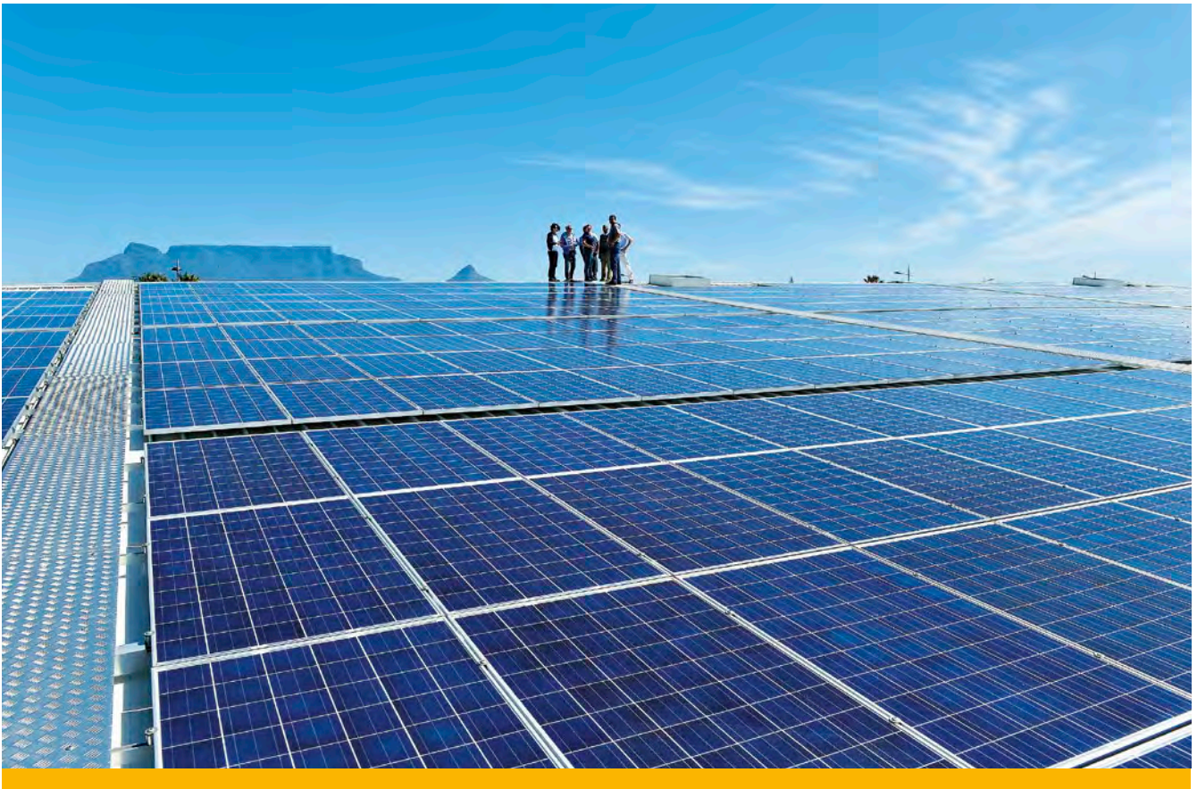
Solar PV panels on Bayside Mall. Photo credit: Bruce Sutherland, City of Cape Town.
